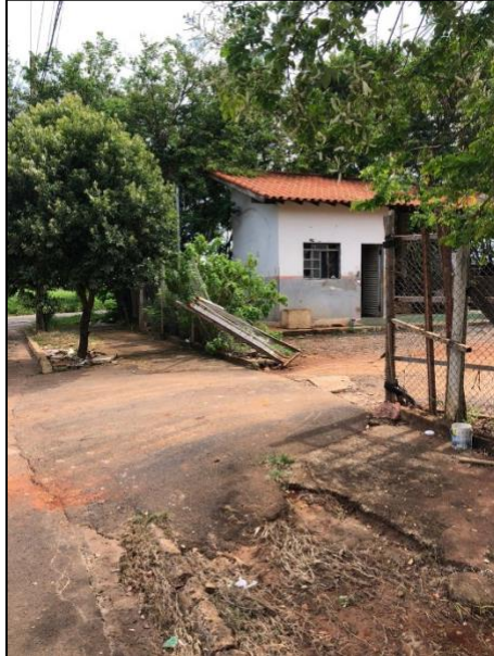
Figure 5. Entrance gate to ecopoint 3 in poor condition
